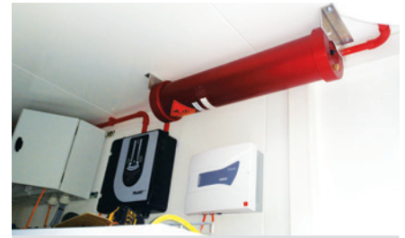
Typhoon® Fire Suppression Equipment installed horizontally (ceiling mounted)
